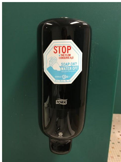
Figure 5: Signage in their restroom as a reminder to turn off the water while soaping your hands
