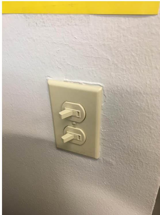
Figure 3: Current office light switches that do not have signage to remind office members to turn off the lights when they leave the room.
