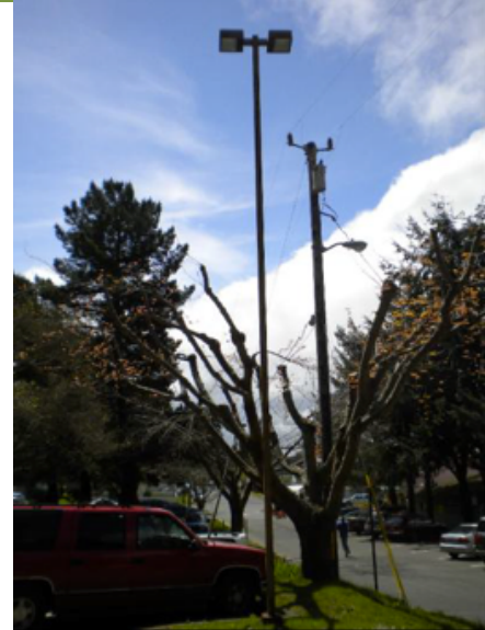
The existing High Pressure Sodium pole in 14th Street Lot
