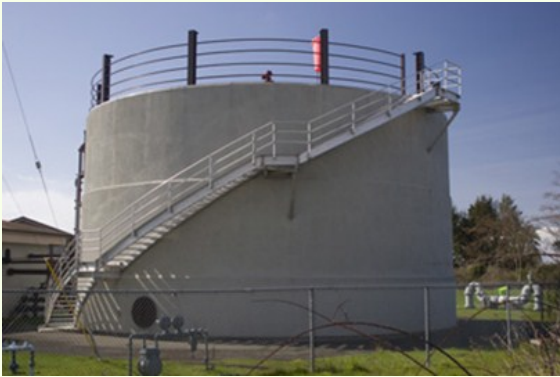
ABOVE: Digester at the Arcata Wastewater Treatment Plant (Poppendieck, 2008)
