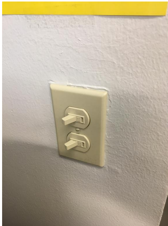
Figure 2. Current office light switches that do not have signage to remind office members to turn off the lights when they leave the room.
